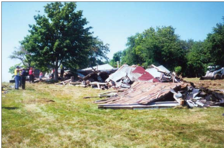
Fig. 93: Several of the cottages were demolished in July 2001, including Cottages 8, 9, and 10 on the south side of the island, above. (Claire Pierimarchi Hale)
